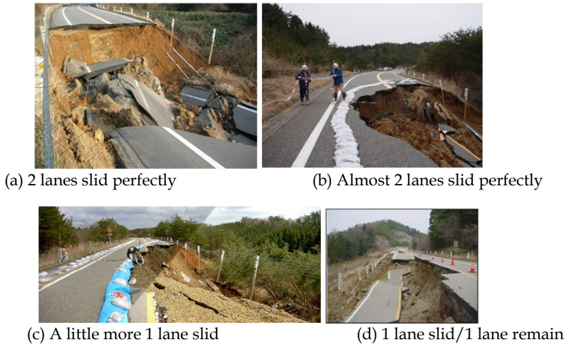
Photo 3. Large-scaled damage of road embankment without traffic performance
