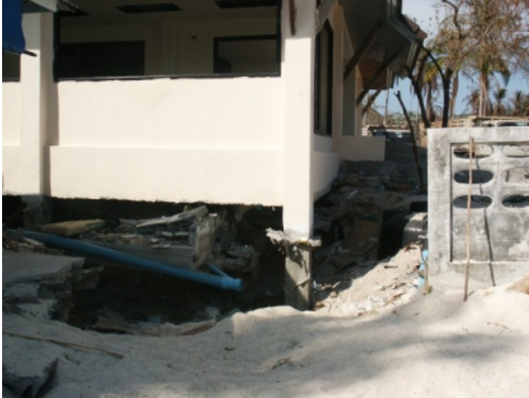
Fig. 40. Scouring of Foundation Soils and Severing of Building's Utility Lines, Phi Phi Island Hospital, Thailand, 2004.
