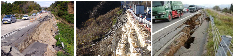
(a) Partial sliding and urgent retrieval with sand bags
