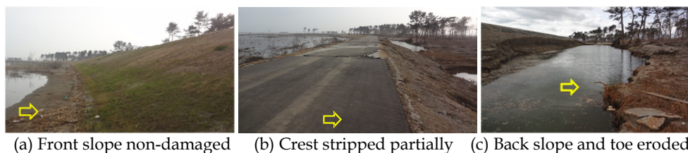
Photo 8. Dyke overflowed by tsunami
