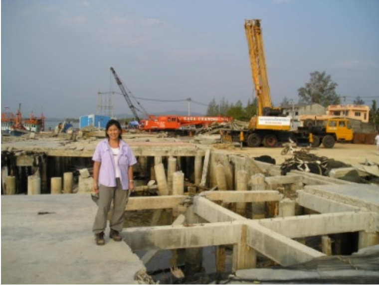
Fig. 36. Wharf Damaged by Wave Impact and Uplift, Bam Nam Kem, Phang Nga Province, Thailand, 2004.
