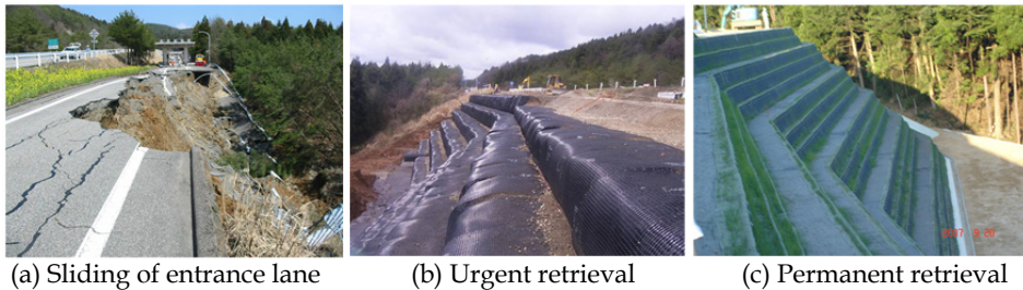
Photo 4. Damage and seismic retrieval with geotextile
